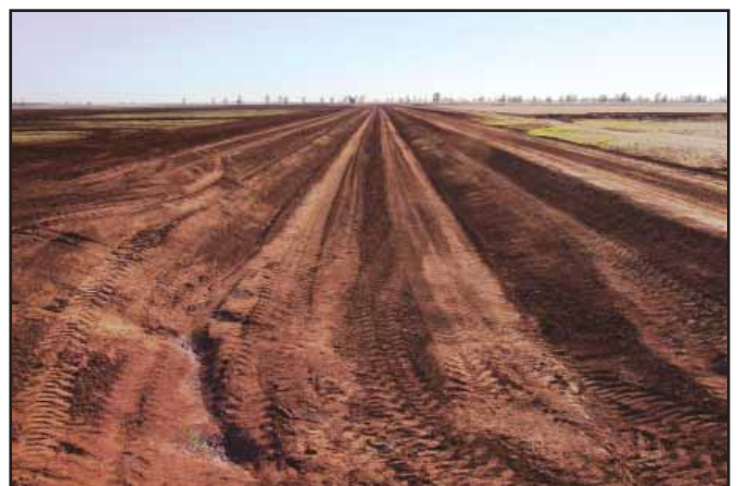
Figure 3: The new diversion channel built to prevent further spread of alligator weed
