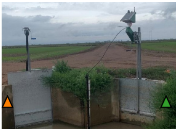
Manual sluice v Automated sluice
