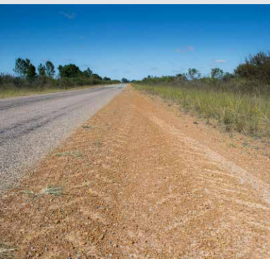
A typical minor bitumen road in cropping areas of Western Australia. AGRONOMO
